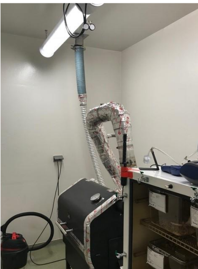
Figure 1. Electric smoker connected to central exhaust system
